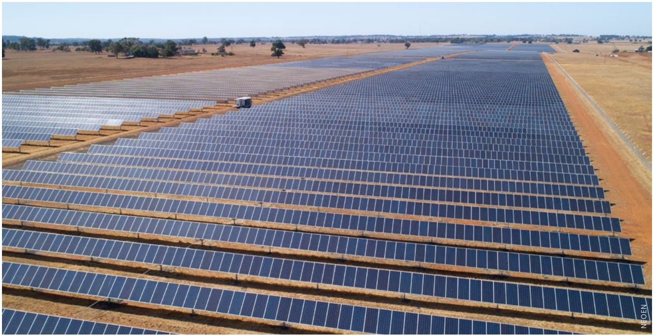
^ The 28-MW Dubbo Solar Hub was completed in 2018 by Neoen in Australia.
